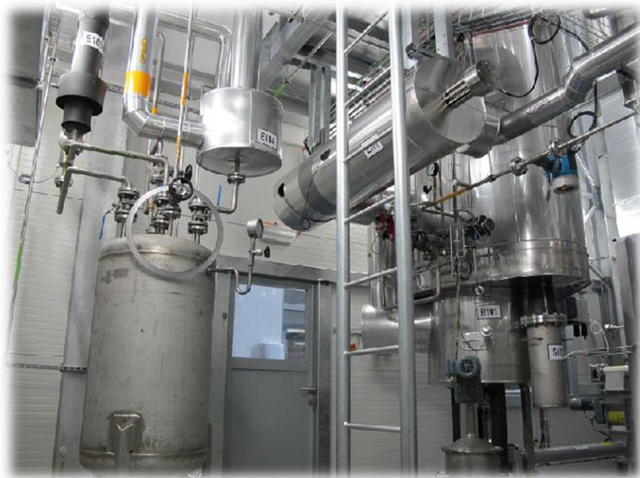
Bottom section with fuel transport (right side)
